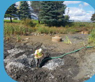
Phase II, a fully drained portion of the system
